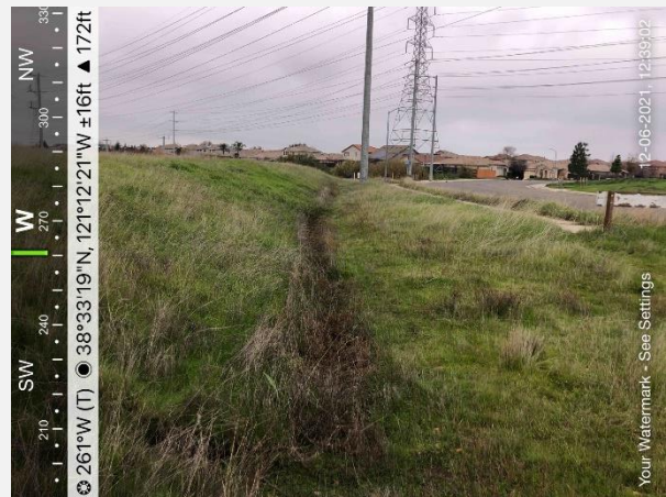
Photo 14. Stormwater control feature along the northern boundary of the PSA.
