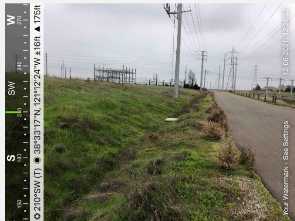
Photo 16. Stormwater control feature along the western boundary of the PSA.
