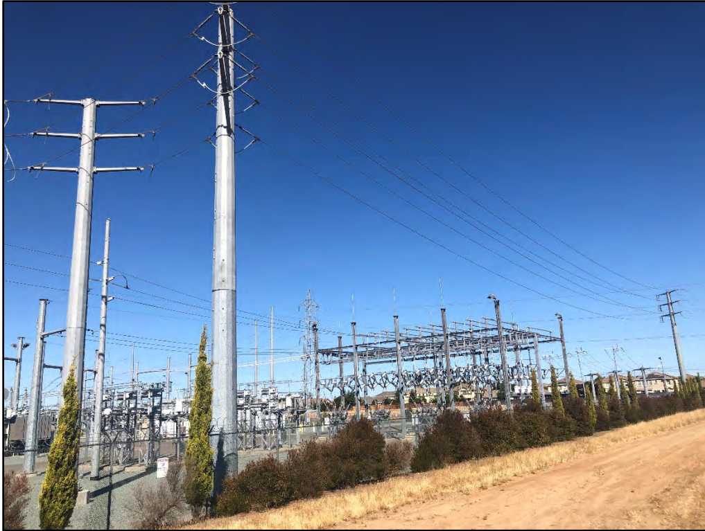
Photograph 1: View of the switch yard on the southern side of the subject site.
