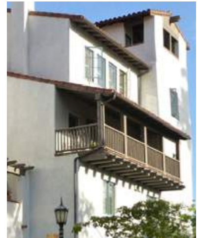
Balcony Overextending Sidewalk
