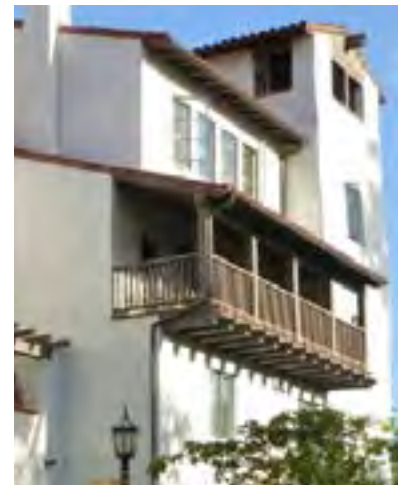
Balcony Overextending Sidewalk
