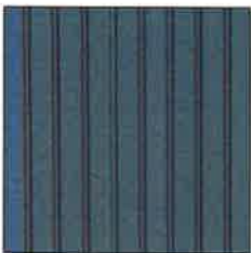
TEAL OCCURS AT CEMENTITIOUS SIDING
