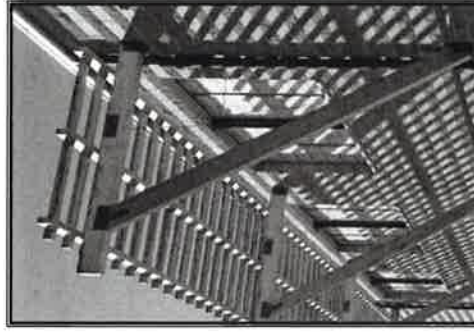
This trelliswork allows some light to flow to the building windows, but filters the overall amount. The intended results include reducing the impact of solar heating on the building, thereby reducing overall cooling costs. It is also an attractive architectural feature of the building (Courtesy LPA)
