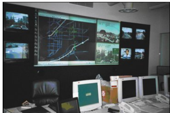
Figure 21 – Sacramento County Traffic Operations Center
