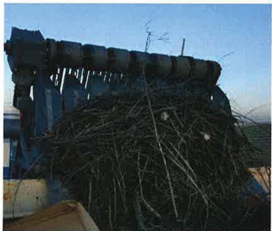
Photo 2 - D-44 Bear Hollow Trash Rack filled with Branches from Beaver Activity in Basin
