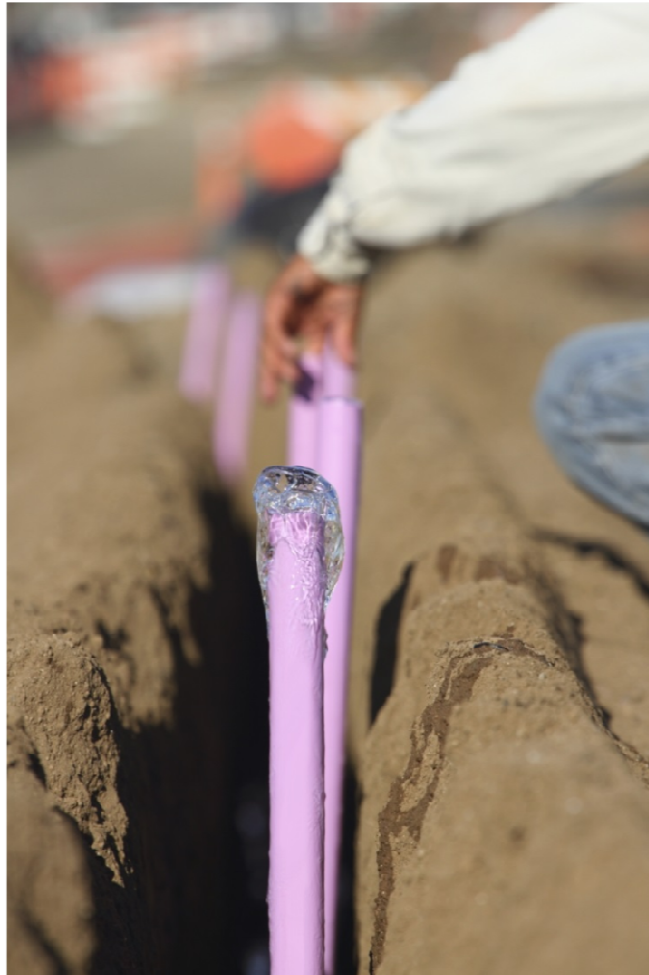
Reclaimed water is distributed in purple pipes to distinguish it from potable water
