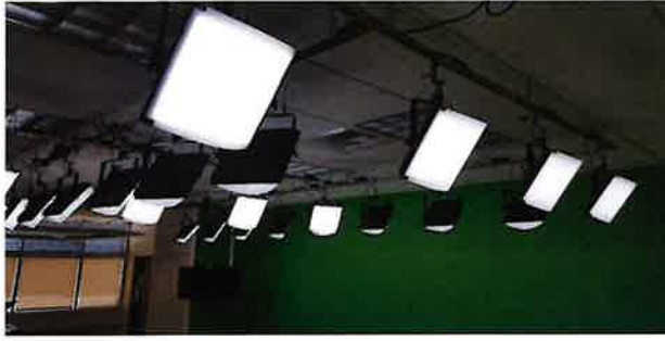
Example Photo of LED lights attached to unistrut
